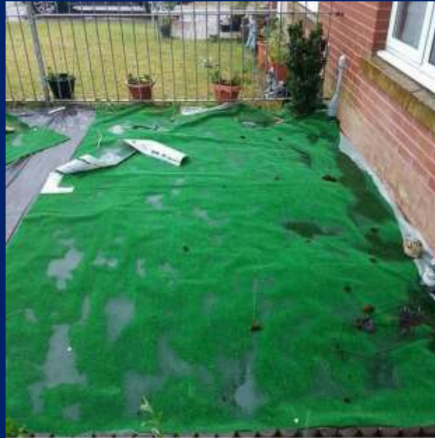
Site Drainage Issues
